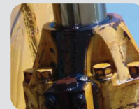
Seal Damage, Leaks
